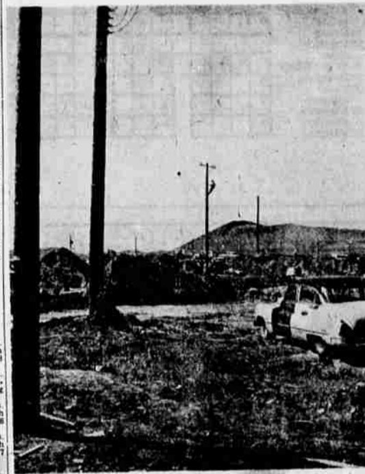
POWER POLES AND EARTH MOVING on the Miller Hill site of 290 homes signify the preparation necessary to get new home sites ready. The Gresham-Alcan Company is moving at full speed with a contract that calls for over 4 million dollars in construction between now and early spring 1959. The initial contract for 220 homes was for $3,484,622, and later another contract for 70 additional homes was signed for the same area in the amount of $1,155,000. — Photo by Kettler
