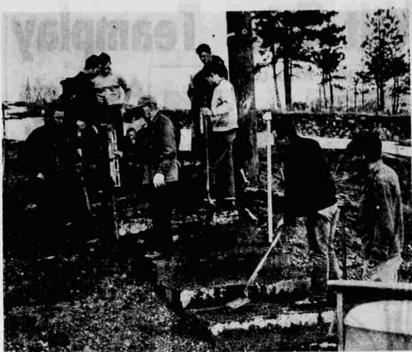
DIESEL ENGINEERING can become pretty diversified. Here, members of the diesel engineering class take on the project of rebuilding concrete steps up to the girl's dormitory at Oregon Tech. In the foreground are, left to right, Jerry Dittbenner, class president; Merle Jackson, center with level, and Fred DeWitt, lower right with shovel, instructors; and extreme lower right, Don Vander Zanden, student. Other diesel engineering students are shown in the background as work progresses on their rebuilding project.
