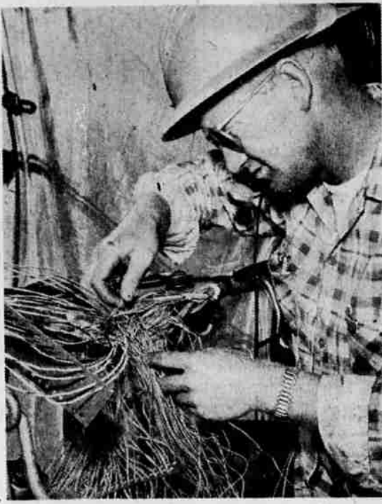
PERCHED ALOFT on an aerial platform, Pacific Telephone splicer, M. A. Dorman, 2732 Summers Lane, connects wires from four cables together in one of seven cable projects being completed in Klamath Falls area by the company this year.
