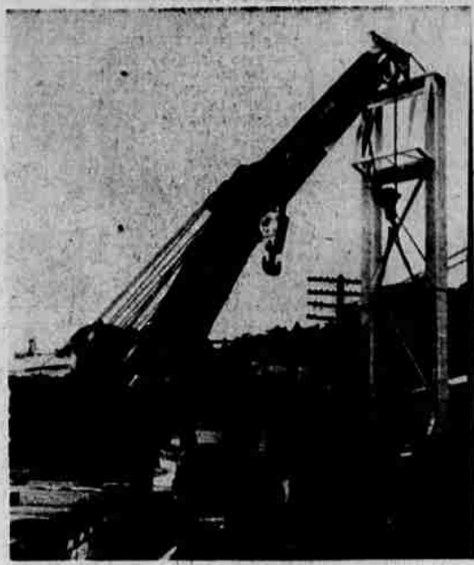
MICROWAVE TOWER AT DUNSMUIR being lifted into place by Southern Pacific's giant crane, part of a microwave installation to insure more dependable communication between Shasta Division headquarters and Black Butte. — Photo by Thelma Thoreson
