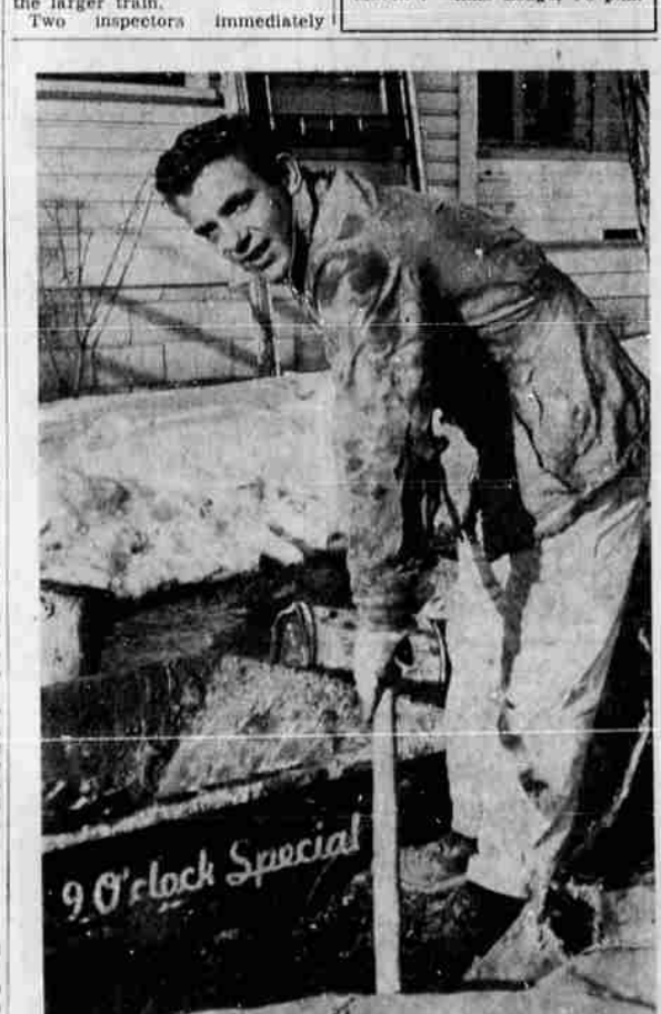
DICK JONES, 3407 Bisbee Street, was hard at work this morning when interrupted by the 9 o'clock photographer. Jones is an employe of Lou Hatfield, masonry contractor. The work was in progress at a house on 512 North Ninth Street.
