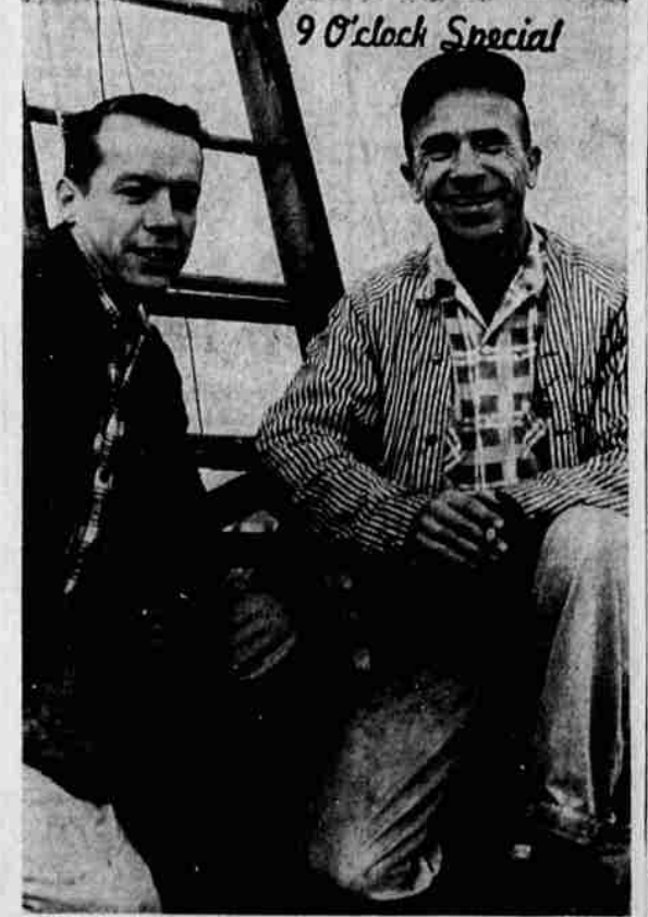
J. E. JOHNSON, LEFT, AND Don Strupp , employees of the Oregon State Highway Department, were caught by the 9 o'clock photographer this morning as they were repairing the blinker signals on the Sixth Street overpass. The two men, residents of Grants Pass, are on roving assignment status with the department.
