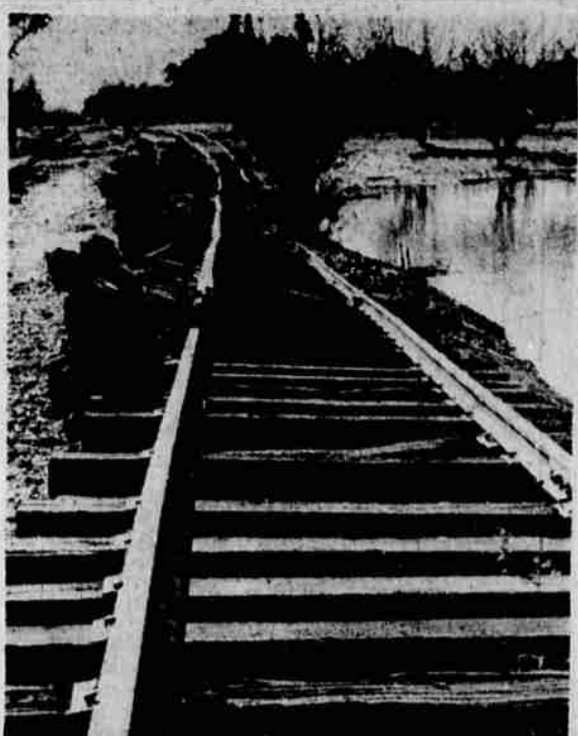
TRAINS WERE HALTED for several days in the Yuba City, California, area, when flood water from the Feather River undermined right of ways. Don Kettler, Herald and News photographer, obtained the above picture of the stretch of track twisted out of shape by the flood.
