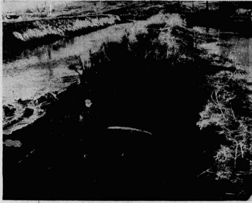
TORRENTIAL RAINS Wednesday night and Thursday caused miniature rivers to roar down the hillside above the A Canal and caused this break in the canal bank. A small water main of the Oregon Water Corp. was broken as a result of the cave-in. The break occurred on Alameda Avenue beyond the city limits. Wallace Milligan, Oregon Water serviceman, is shown at work on the break Thursday. The service was restored Thursday.
