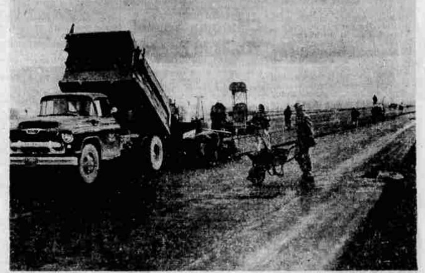
RUNWAY CONSTRUCTION is proceeding at a fast pace at the new Klamath Falls U.S. Air Force Base. In the upper picture the mixing plant, operated by the D-H Paving Company, Portland, is turning out the asphalt mix which is trucked to the runway.
