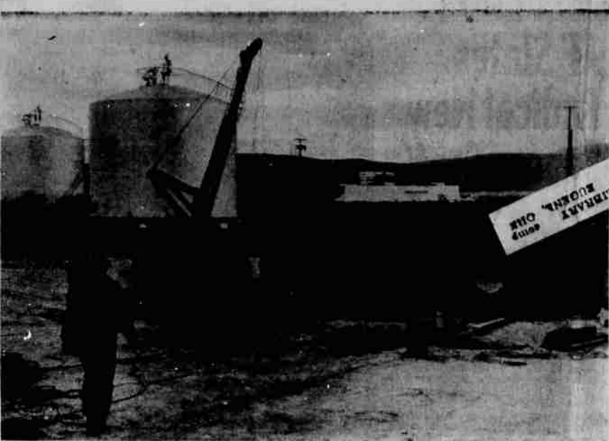
NEW JET FUEL STORAGE TANK at the Klamath Falls Air Force Base is being constructed by crews of the Hammond Iron Works, Salt Lake City. The tank is being built near the existing fuel tanks built by the Navy during World War II.
