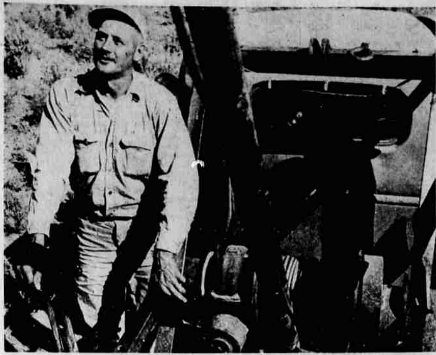
RALPH WHITE, operations foreman of Carlson Construction Company, handles the boom truck winch to hoist one of the last 537 poles of the 69 kv transmission line into place to bring rural electrification to north Lake County. The new 150-mile system will be energized following dedication ceremonies Friday, October 28, at Silver Lake.
