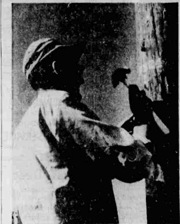
JOHN A. UNFRED, partner of C. W. Brown of the Northern Construction Company which has built 150 miles of line for an electrical distribution system in north Lake County basin, is shown tacking on final pole numbers. —Photo by Parks
