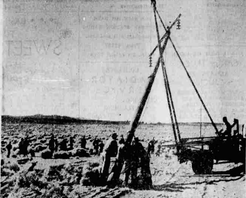
PUPILS of the Fort Rock School watch a power pole being raised by a Carlson Construction Company crew for the 69,000-volt main transmission line crossing the old Dave Busch place near Fort Rock. School boys helped tamp the dirt around the pole after it was set. This is part of the project of bringing electricity to the Fort Rock and Silver Lake area.
