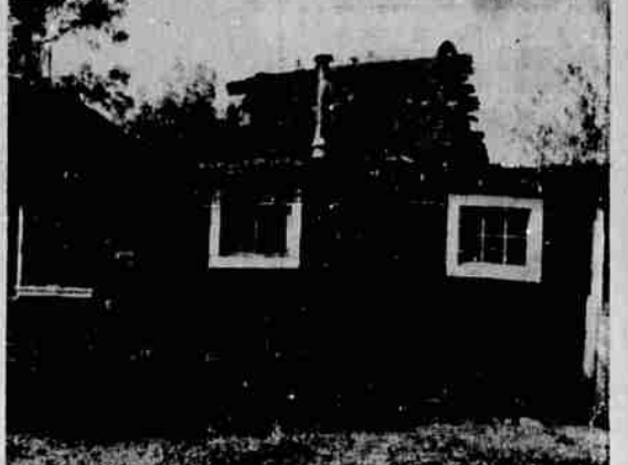
A STOVE EXPLODED in this two-family dwelling in Weed at 6:40 a.m. Thursday, completely gutting the building. Two families, each having three children, lost all personal belongings. Burned out were the families of Paul Painter, Long-Bell Lumber Company employe, and Frank Morrison who is employed at the Medo-Land Dairy near Weed.
