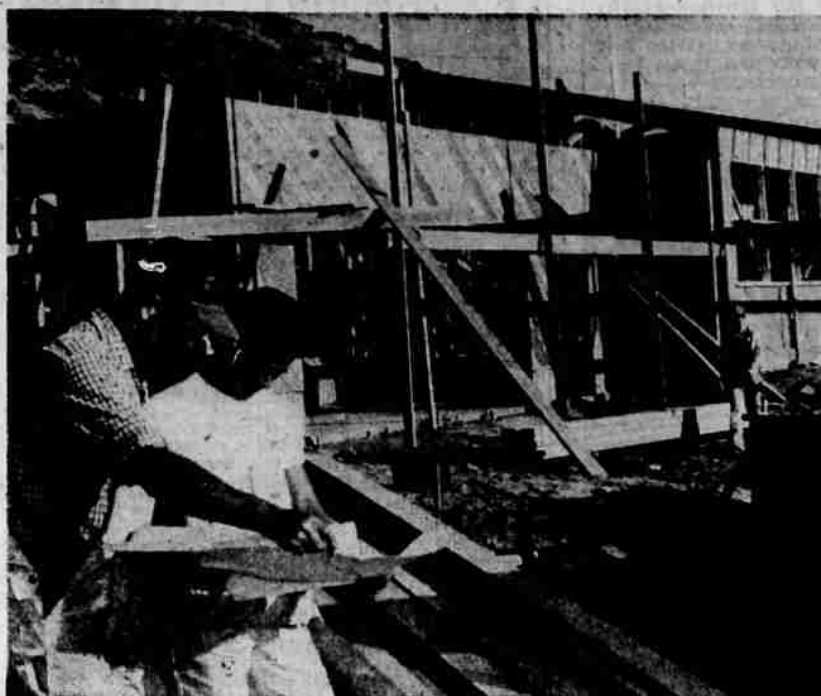
A NEW HOME now under construction in the Hot Springs district is being built for Dr. John Merryman on Fairmont Street. Shown checking plans are Norman Jones (left) and David Jones. Contractors are Norman and Bill Jones.
