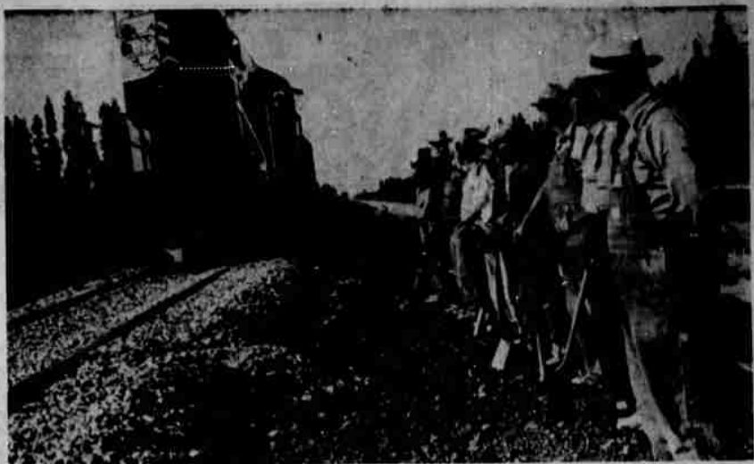
FACE-LIFTING of the Great Northern tracks in the La Pine area is under way this season, changing the Klamath Division's 68-mile "north end" from 70-pound rails on cinder ballast to 115-pound steel laid on uniform well-drained crushed rock. Rudy Zlatich and his gang are shown standing in the clear while a freight train eases over rock ballast dumped only a few hours before. — Photo by Helen Parks, Fort Rock.
