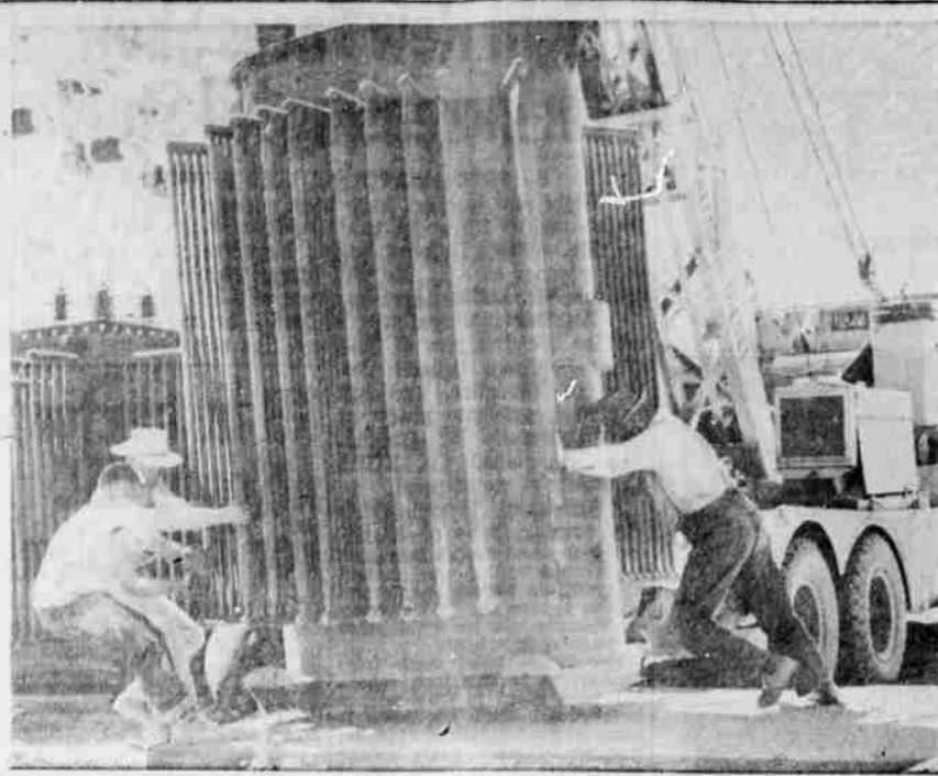
HUGE TRANSFORMERS for the new power lines to connect LaPine and the Fort Rock, Silver Lake and Christmas Lake area, were recently unloaded by a crew including the men shown, from left: Bob Gilder, Pat Allison and E. J. Williams. Leon Gilder, Bob's father, supervised the spotting of the transformer. —Photo by Helen Parks
