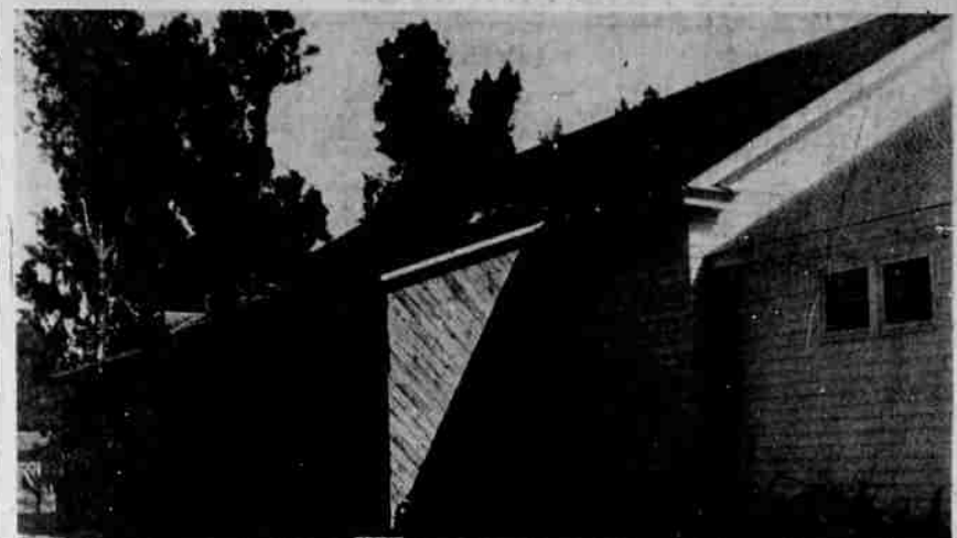
CONSTRUCTION IS NEARING completion on the new seating arrangements being built on to the Malin High School gymnasium. This addition is expected to seat an additional 510 spectators.
