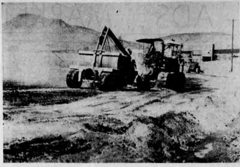
THE GROUNDWORK FOR the new home of the Klamath Irrigation District is nearing completion at its new location south of the "C" canal at the "C" canal power plant in the Henley district. KID is using its own equipment to do the fill work.
