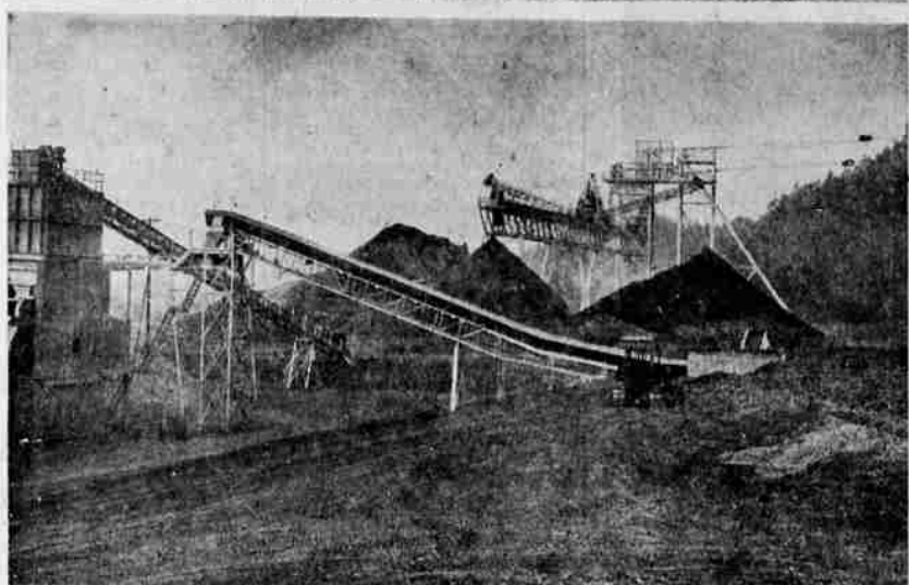
THIRTY MILLION DOLLAR SOUTHERN OREGON DEVELOPMENT — These two pictures illustrate sketchily what happens when modern technology and hitherto undeveloped raw material resources come together. The upper picture shows the smelter building at the Hanna Nickel Smelting Company's operation at Riddle, in Douglas County. Shown below is the hogged fuel conveyor that feeds furnaces where the ore is dried. Also visible are ore stacking equipment, a pile of ore in the stockpile grounds and, at left, an end view of the ore reclaiming tunnel. The ore comes from Nickel Mountain, a mass of low-grade nickel ore at the edge of the town of Riddle. New processes have made its development possible. A total of some 30 million dollars is being spent in the project. A new development of similar magnitude for the Klamath Basin is possible through utilization of jackpine, formerly regarded as useless, but now recognized as one of the most valuable pulp woods in the West.
