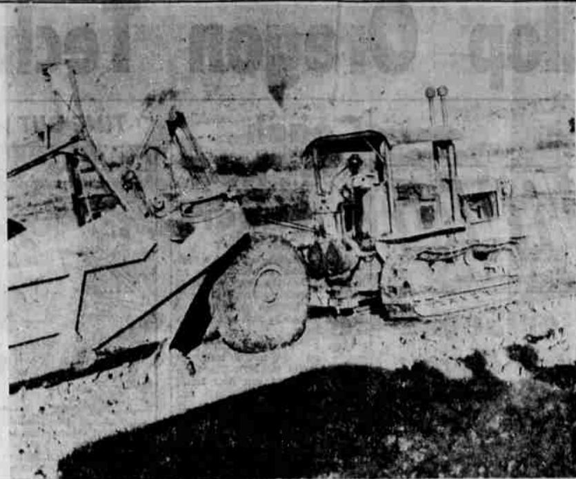
THIS IS HEAVY EQUIPMENT being used to level ground on Shasta Way for a business and shopping center. Ten acres of land will be included in the project owned by John Fehlen, 3803 Frieda Street.
