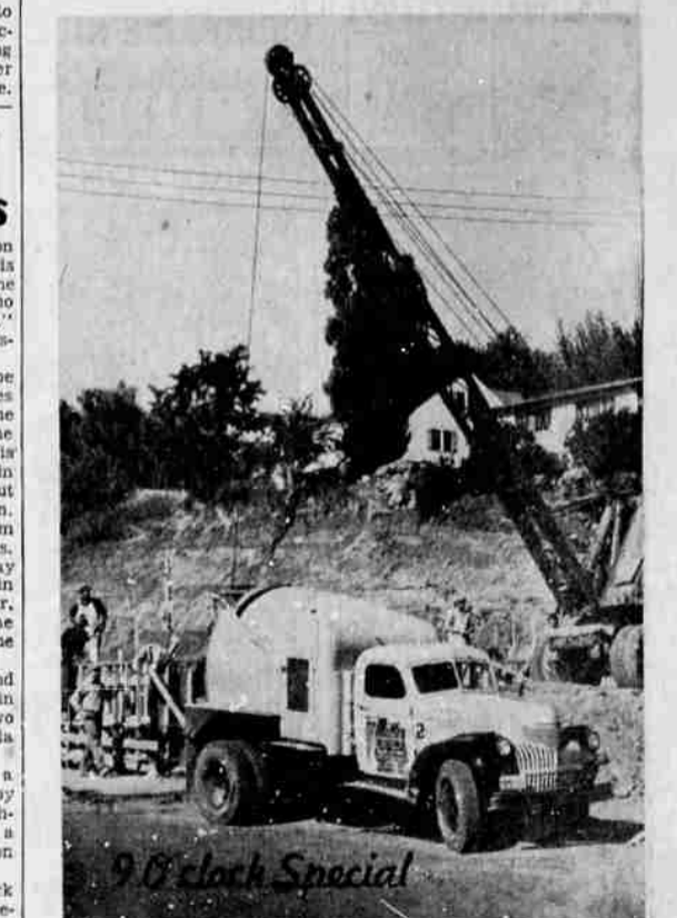
CONCRETE WORK ON new motel site at 75 Main was the topic of the early morning photographer this morning. Completion of the motel is expected by the first of the year according to the owners, Mr. and Mrs. C. C. Nelson.
