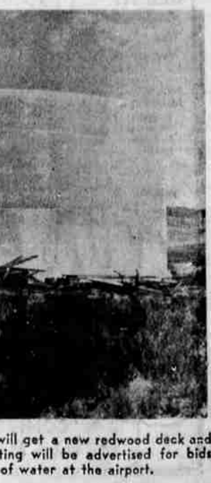
THE MILLION GALLON STEEL WATER tank at the airport will get a new redwood deck and built up roof now; necessary sandblasting, scaling and painting will be advertised for bids this fall. Action was speeded to prevent possible rationing of water at the airport.
