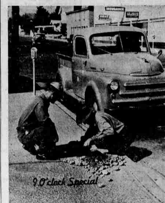
LOOKING FOR A PENNY? No. They're relocating a parking meter on Seventh and Pine which was set in cement Tuesday, bumped by a passing motorist Tuesday night, and just a hole in the ground Wednesday. At left is Al Brotherton, city meter maintenance man, with A. J. Landrie, city street employee.
