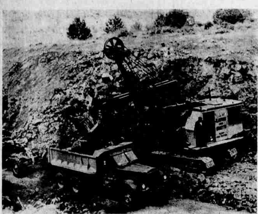
HEAVY EQUIPMENT BITES INTO THE DORRIS HILL as work progresses on the widening and sloping of the deep cut in an effort to eliminate the icy condition of the roadway during the winter months. The hill has long been considered one of the worst on Highway 97. Eaton and Smith, San Francisco, are the contractors.
