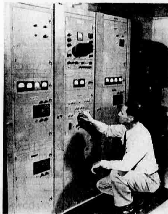
A COMPLEX MAZE of wiring and instrument panels confronts the engineer when he gets into Omrange, the new navigational aid just established at the Klamath airport. This new aid to flying replaces the old four-course directional beam and allows a pilot a 365 degree range in selecting courses between Omrange stations.
