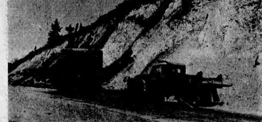
OREGON STATE HIGHWAY CREW cleans up the sides of Highway 97 north of the city limits from the effects of the winter slides.
