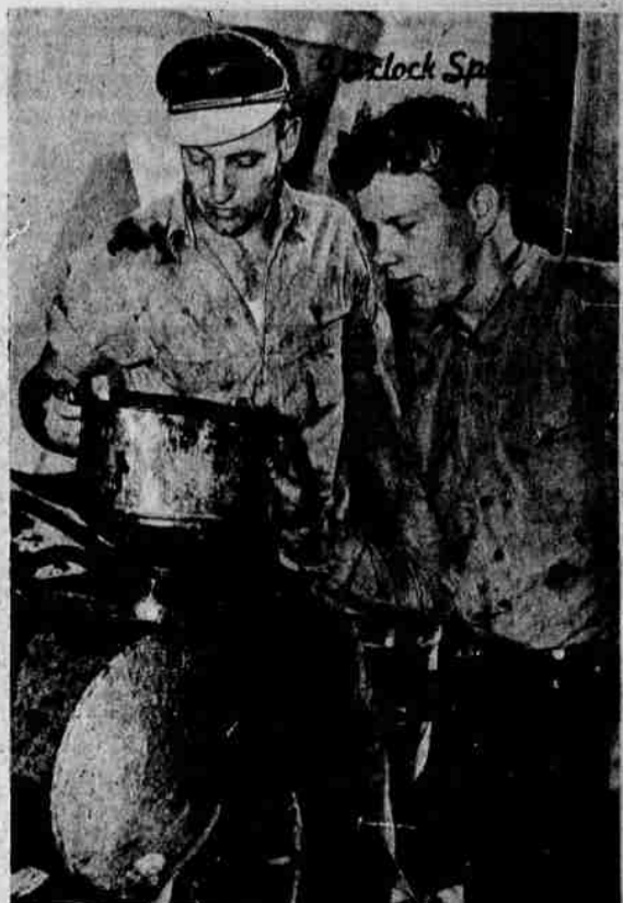
FILLING UP THE TANK this morning before starting a roofing job at 1330 Main street was D. R. Phillips and Kenneth Ducat.
