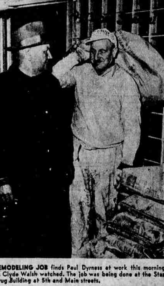
REMODELING JOB finds Paul Dyness at work this morning as Clyde Walsh worked. The job was being done at the Star Drug Building at 5th and Main streets.
