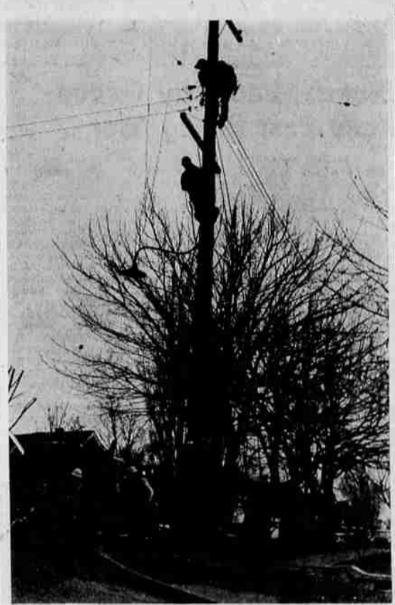
HIGH ABOVE THE GROUND these Copco workers were busy at the corner of Fourth and Jefferson the other day putting in one of the new, taller poles.
