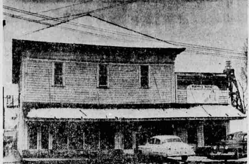
WORKMEN ARE RAZING this old landmark in Merrill, constructed about the time the town began to grow and used for many years as a town meeting place. —Photo by Van
