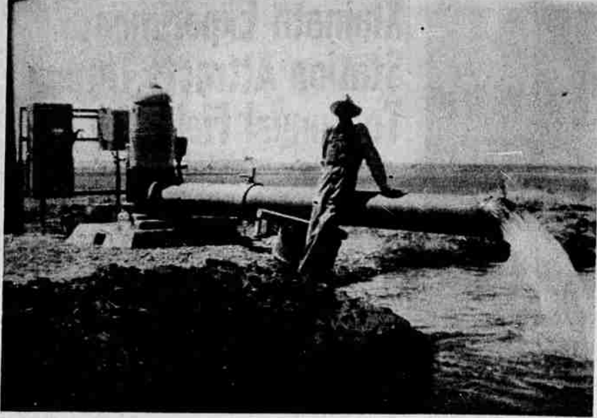
TED JOHNSON'S new well in Butte Valley throws quite a stream of water, as this picture shows. East of Macdoel, the pump discharge of the well is approximately 3200 gallons per minute at a pumping depth of 82 feet. Johnson is bringing 160 acres under irrigation from the well.
