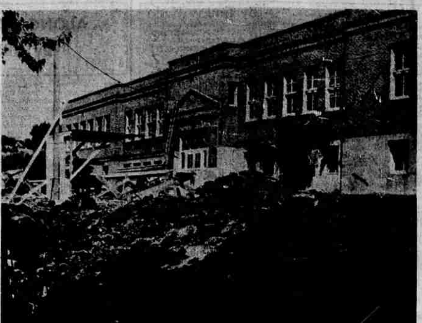
SIX NEW classrooms, a completely rebuilt kitchen and cafeteria, and force ventilation for the entire building are in store for students and faculty at Fairview School. A rock retaining wall on Donald Street is also being built to increase the playground area. Construction time is 200 days and will probably be completed by January 1. Fininger and Watkins are the contractors; Howard Perrin, architect. Construction cost will be $120,000. The exterior is brick.
