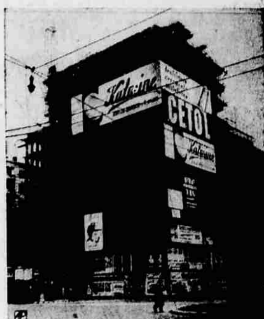
TOWARD EUROPE'S SKIES —Work reaches 11th floor of modern skyscraper being erected in Milan, Italy. Building, reported to be highest in Europe, will have 30 floors.
