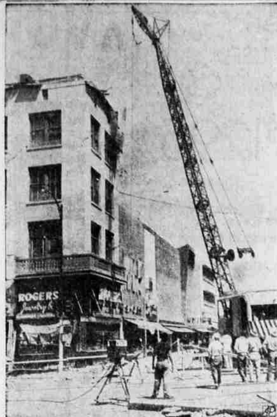
DEMOLITION WORK —Workmen with huge cranes like this one began the work of tearing down unsafe walls of buildings wrecked by the earthquake that shook Bakersfield, Calif., killing two persons and doing millions of dollars in damage.
