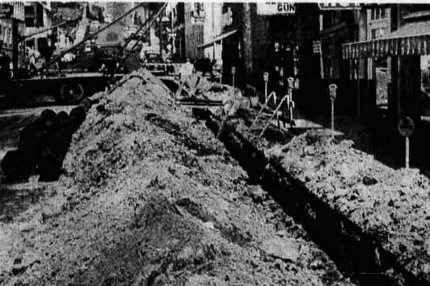
OLD SIX-INCH WATER MAIN pipe is being replaced now with a 12-inch main, accounting for the deep ditch which has been put in S. 6th between Main and Klamath this week. Next Monday the ditch is to be extended across Klamath Avenue and on to Walnut Street.
