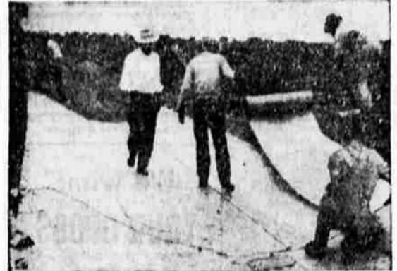
STRIPS of fiber glass are laid like carpets and an asphalt membrane is created by spraying with a hot solution.
