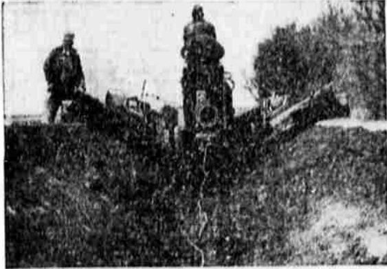
A PLOW-TYPE ditch-digger prepares the canal for lining. Low-cost canal linings in Federal Reclamation projects have saved more than five million dollars in water in the west. So the Bureau of Reclamation has published a booklet on "Canal Linings and Methods," it is available from the Government Printing Office, Washington 25, D. C., for 25 cents. It says water lost on 46 federal projects would have irrigated an additional million acres of land.
