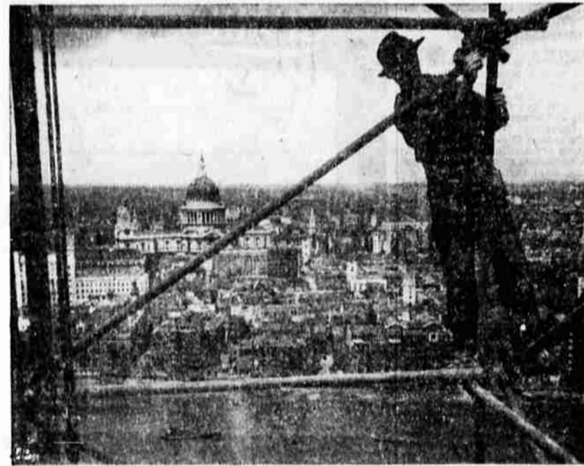
SKY WORKER ON THE JOB —Scaffolder Michael Organ rigs a construction platform on a London power plant chimney overlooking St. Paul's Cathedral and the Thames River.
