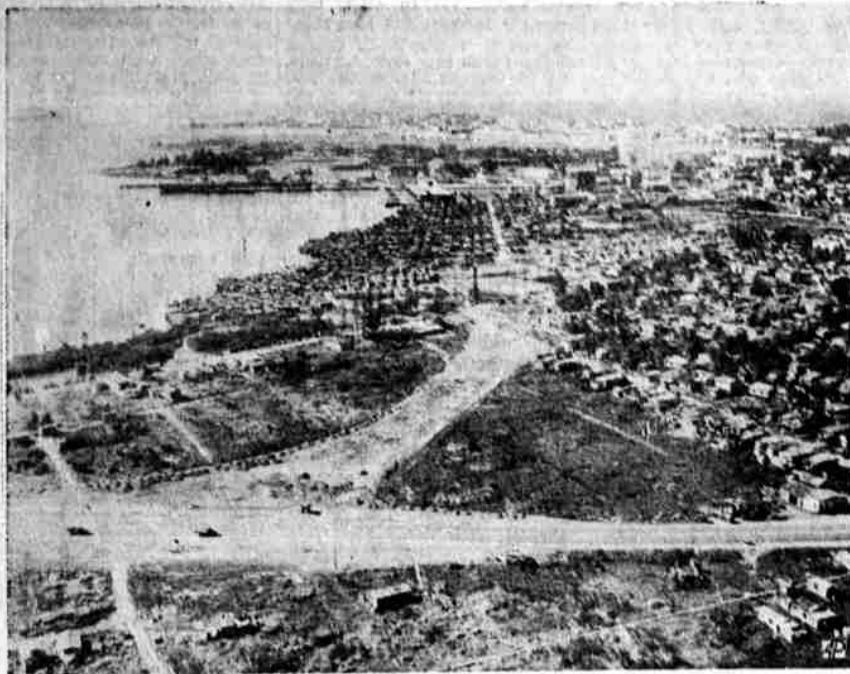
ROAD MARKS PROGRESS — Isla Grande Express Highway, being built on outskirts of San Juan, P. R., cuts through heart of slum area which will be cleared away by end of 1952.
