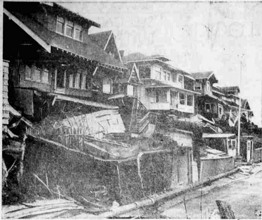
BLOCK BUSTING — This block of homes on Seattle's Queen Anne hill are becoming a jumbled mass of wreckage as continual slides move earth under and around them. The front yards and street have sunk four feet since the first of the year exposing sewer pipe. Two of the homes are still occupied although City Engineering Department expects homes to be completely demolished eventually.
