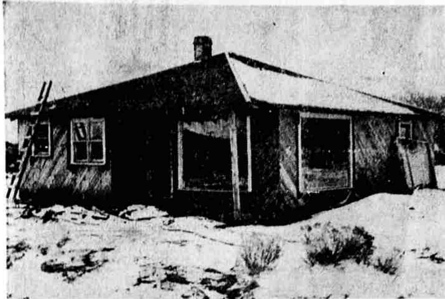
THE LINDLEY STEWARTS of Malin are watching this new home take shape.
