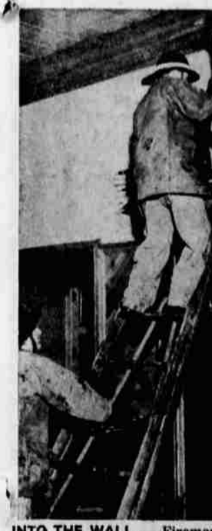
INTO THE WALL —Firemen were called to the pine room of the Elks lodge Saturday afternoon to battle a blaze started in a wall of the lounge room. The fire forced the Elks to shift their Christmas party for children to the armory.
