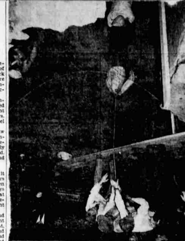
CAVE-IN VICTIM —Rescue workers pull the body of John Cipriani, 30, Monterey, Calif., laborer, to the surface from cave-in where he was killed while working on a sewer construction job at Carmel, Calif. A second man, Carl D. Simon, 25, of Monterey, was also in the cave-in but rescue workers reached him in time to save his life. (AP wirephoto).
