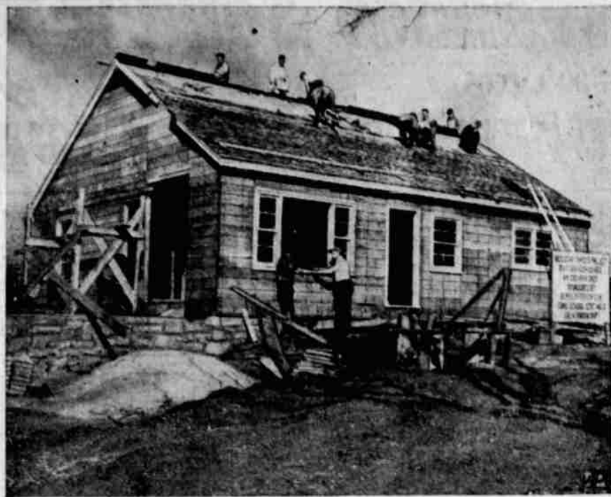
STUDENT PROJECT —Students in the building trades class of Raytown, Mo., High School, work on the six-room house with garage they are building as part of their class work.
