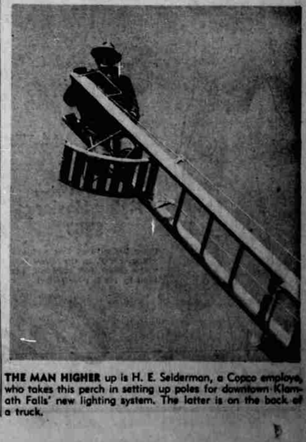
THE MAN HIGHER up is H. E. Seiderman, a Copco employe, who takes this perch in setting up poles for downtown Klamath Falls' new lighting system. The latter is on the back of a truck.
