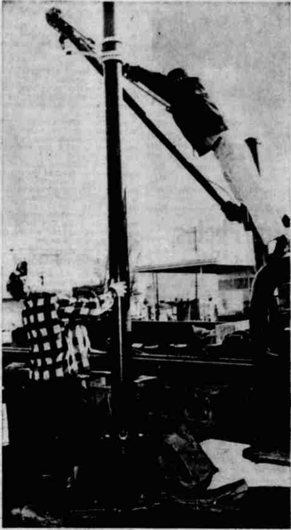
INSTALLATION OF THE new mercury-vapor lights takes a lot of manpower and energy before the 88-unit system can be turned on as evidenced by this action shot of two Coppo workmen on Main street. Frank Nunnally in the plaid jacket watches J. Busick who operates from a power company truck.
