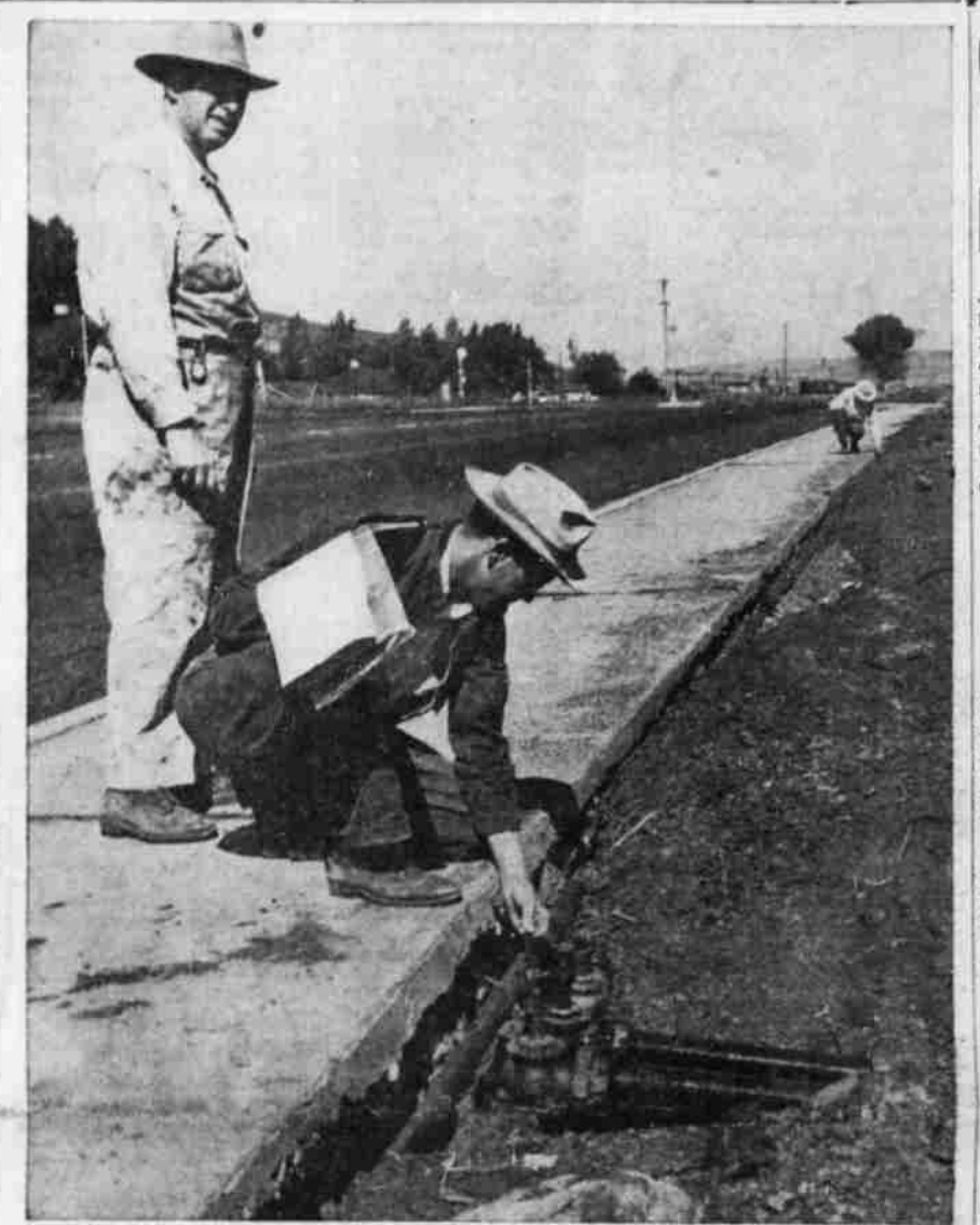
THE JOB OF LANDSCAPING Kit Carson way, known on the maps as the North Entrance, is well under way. Lou Freeman, state highway inspector, is measuring up the pipe job installed this week by C. S. Whitcomb, left, contractor on the landscaping project. Al Tussing, helper, is in the background. The pipes are a part of the sprinkler system which will insure ample water supply for the layout.
