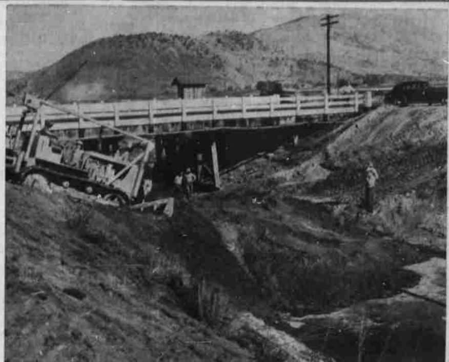
WORKING ON THE DITCH —The bureau of reclamation is widening and deepening the channel of the Lost river diversion canal this summer to raise its capacity from the present 1200 second feet of water to between 2000 and 3000 second feet. Picture shows work being done on the dry ditch where it is crossed by the Merrill highway at Henley.
