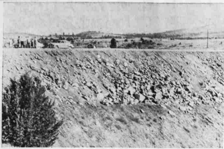
US 395 Improvement—Photo shows construction of fill on new portion of US 395 directly east of Willow ranch, part of a general construction project on this route between Alturas and Lakeview. When completed, probably in 1952, the entire route from Alturas to the Oregon line will have a maximum 3 per cent grade, 100-foot radius curves and 32-foot surface. Last week-end, 15 carloads of road enthusiasts toured the section and had a picnic at New Pine Creek.
