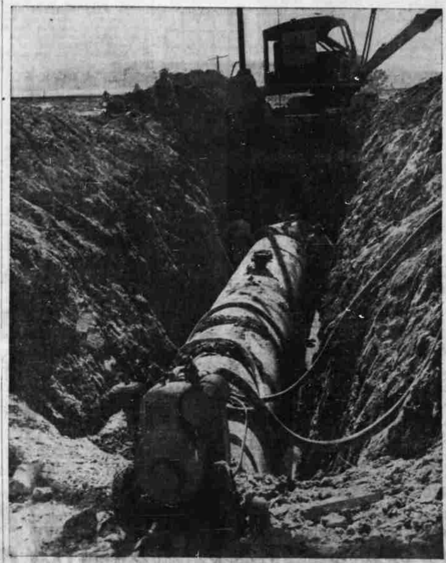
MERRILL ROAD JOB—Workers are shown setting a section of a 48-inch concrete pipe which will carry drainage water under highway 39 at the Wang corner north of Merrill. The highway is being straightened at this point as part of a general widening project now under way from the Seman ranch south. A drainage ditch, part of the farm irrigation system, crosses the highway at the Wang corner and the big pipe is part of this system.
