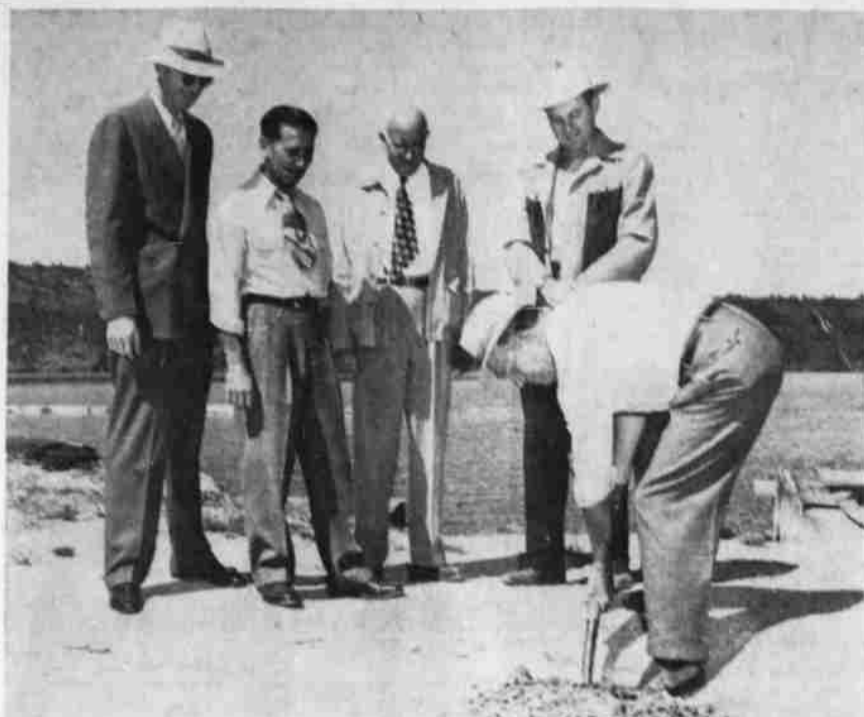
FIRST SHOVELFUL OF EARTH is turned by Mayor Bob Thompson for construction of the Klamath Yacht club building on Front street, facing Upper Klamath lake. Members of the newly formed yacht club watching the proceedings are left to right: Jerry Thomas, Art Rickbeil, Jim Burness and Don Sloan. The mayor is digging.
