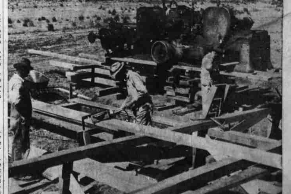
PLANER GOING IN—An eight-knife planer (rear) is being installed at a planing mill being built now by the Ellingson Lumber company on property purchased from the city of Klamath Falls and located on the Great Northern tracks near Memorial cemetery.
